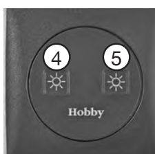
Remote controls, washroom
