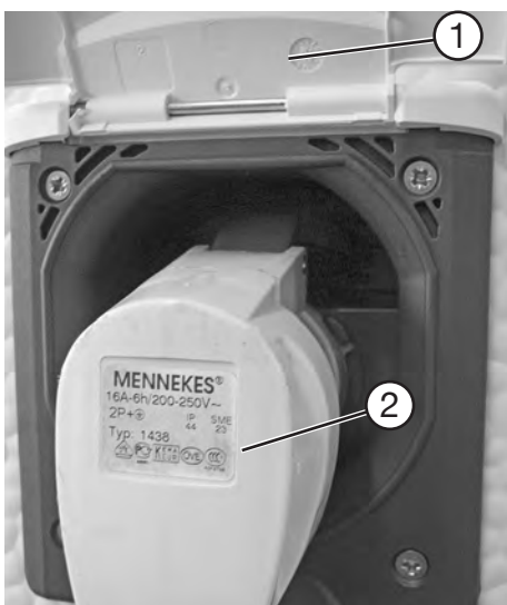
Connected 230V feeder plug
