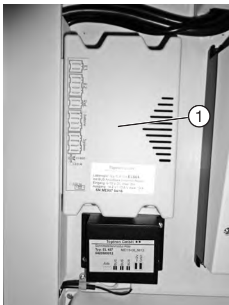
Battery charger ① in the clothes cupboard
