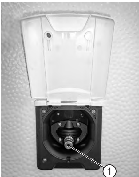
City water supply connection
