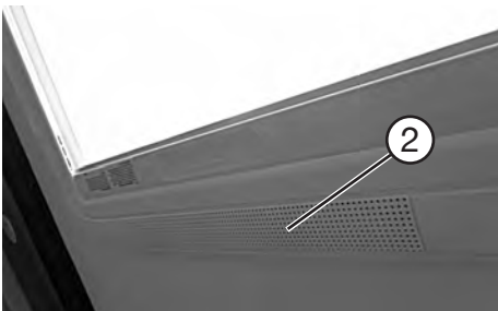
De-aerating via the roof bonnet
