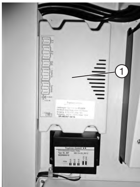
Battery charger ① in the clothes cupboard
