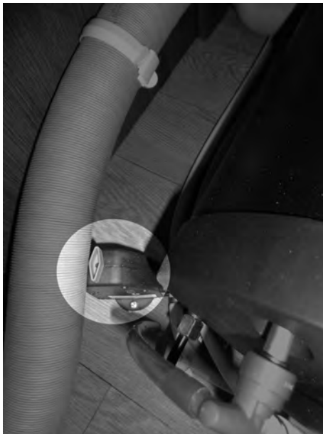
Frost Control valve
