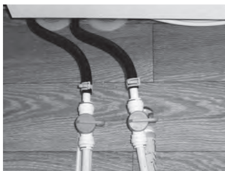
Valves in closed position
