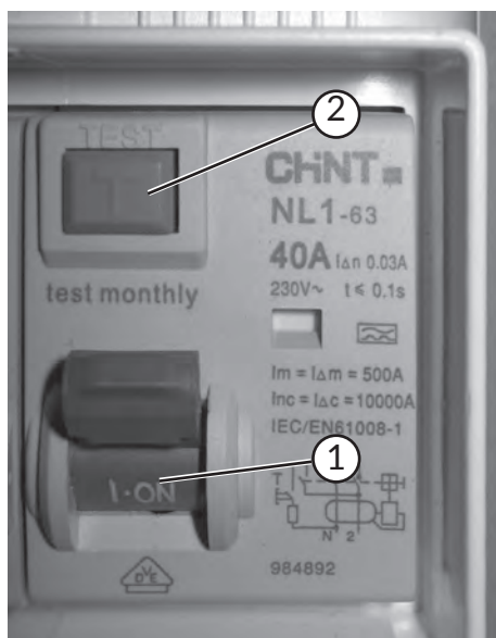
FI switch and test button
