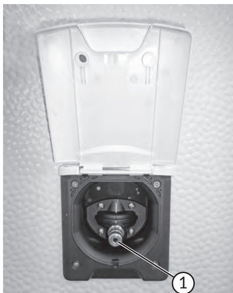
City water supply connection
