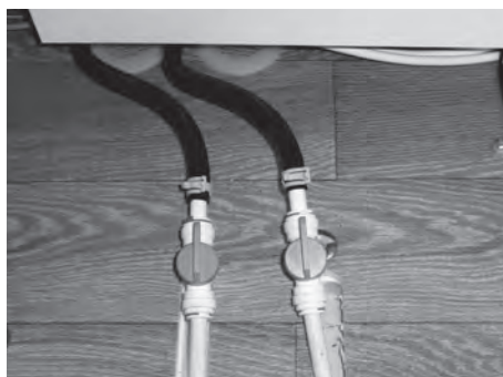
Valves in open position
