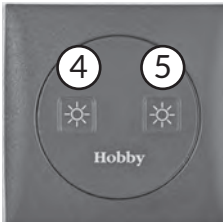
Remote controls, washroom
