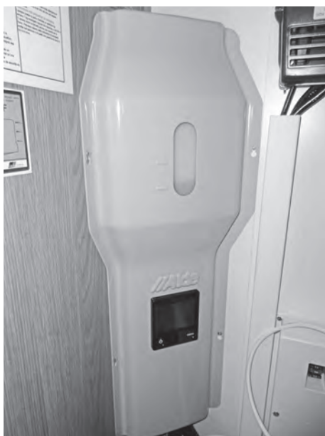
Installation position in the wardrobe
