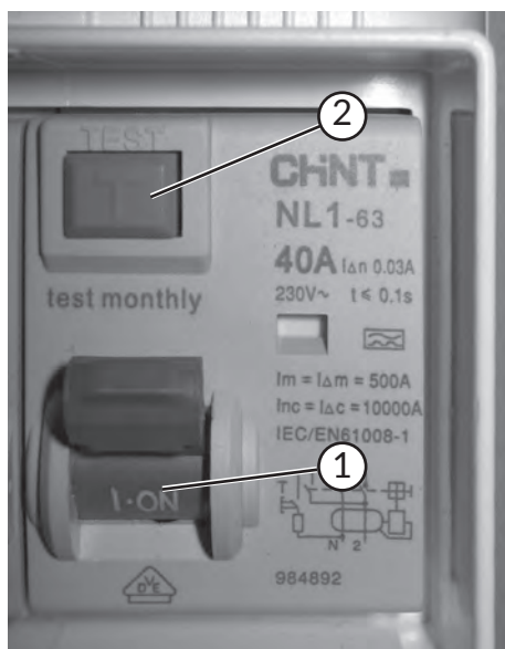
FI switch and test button
