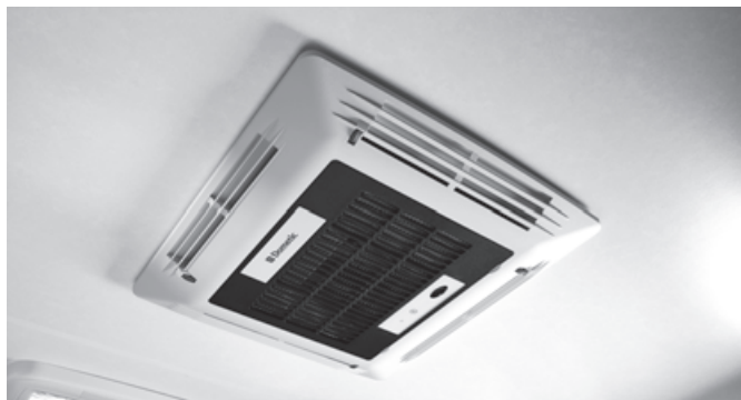
Rooftop Air Conditioning
