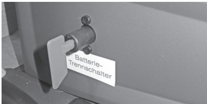
Battery circuit breaker
