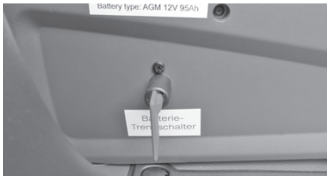
Battery circuit breaker
