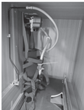
Gas box connections
