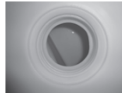
Fresh water tank
