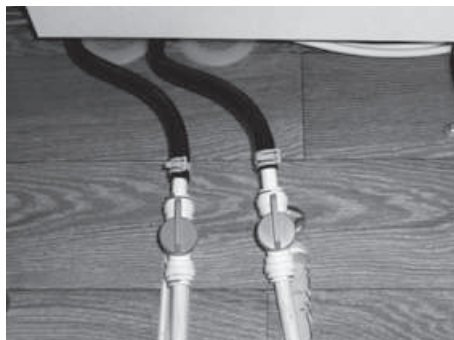
Valves in open position
