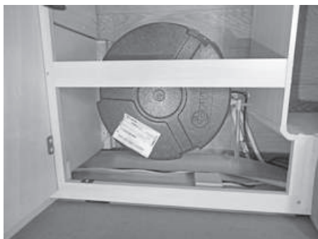
Boiler with drain valve
