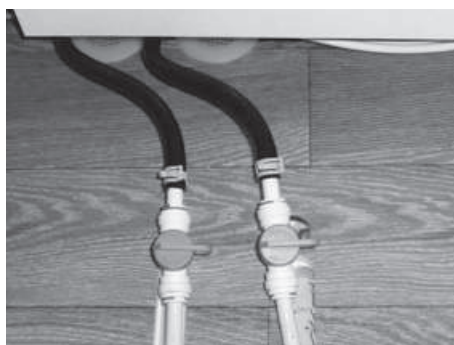
Valves in closed position
