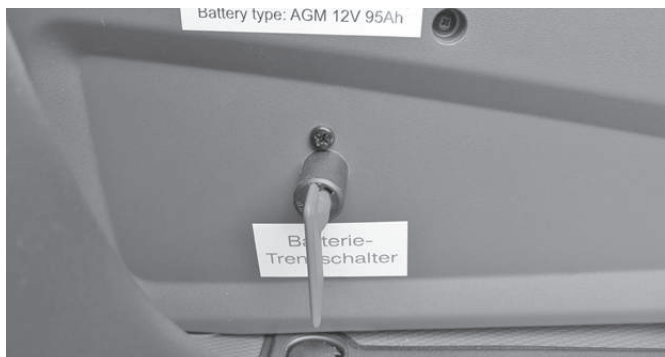
Battery circuit breaker
