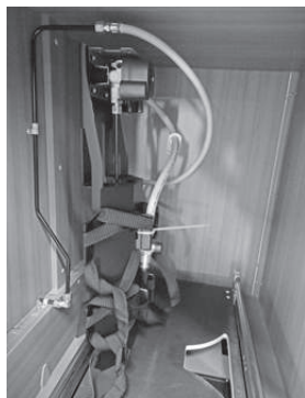
Gas box connections
