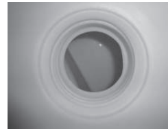
Fresh water tank
