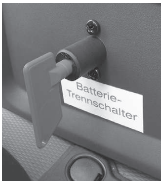
Battery circuit breaker
