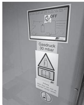
Safety instructions in gas bottle container
