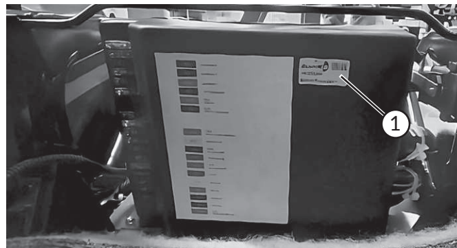
Central control panel with QR code
