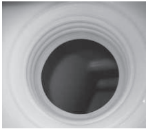
Fresh water tank
