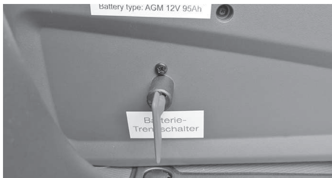
Battery circuit breaker
