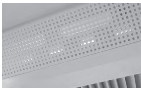
Forced ventilation of the roof bonnet
