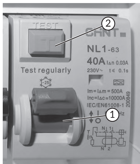
FI switch and test button
