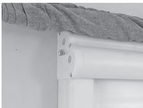
Retightening the tension spring on the shade
