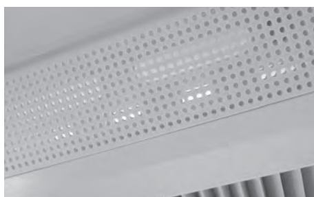
Forced ventilation of the roof bonnet
