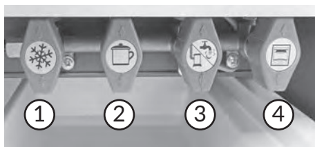
Gas stop valves
