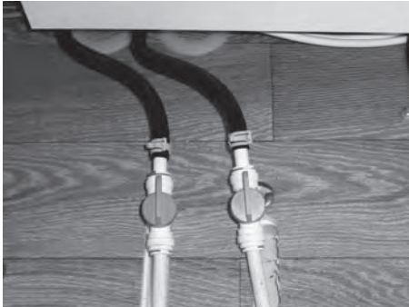
Valves in open position
