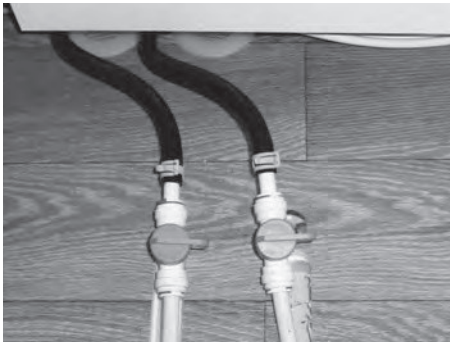
Valves in closed position
