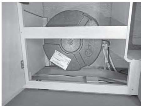
Boiler with drain valve
