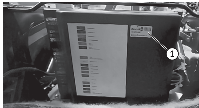
Central control panel with QR code
