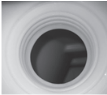
Fresh water tank
