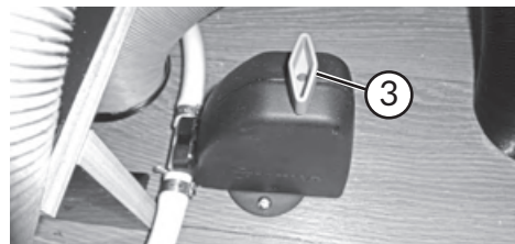
Safety valve for boiler (Frost Control)
