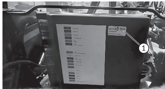
Central control panel with QR code
