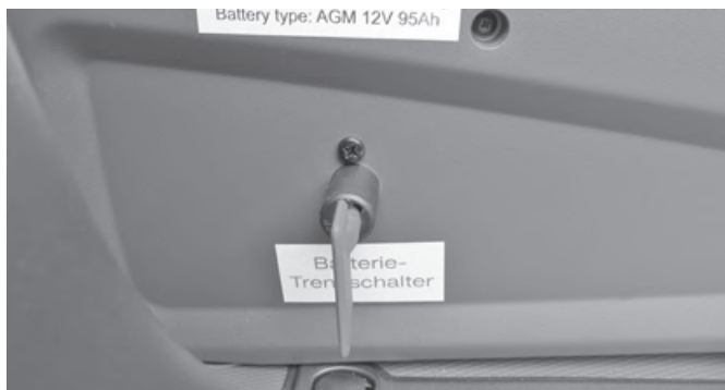
Battery circuit breaker
