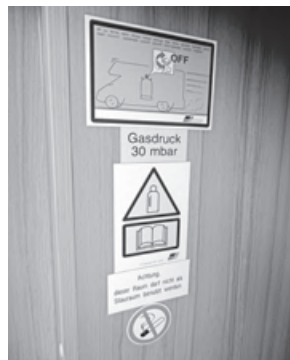
Safety instructions in gas bottle container
