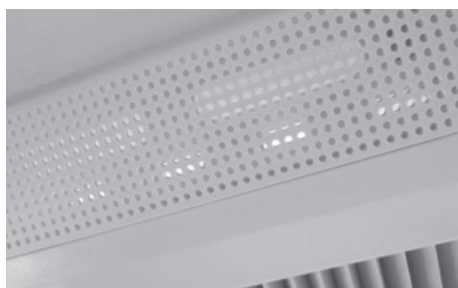
Forced ventilation of the roof bonnet
