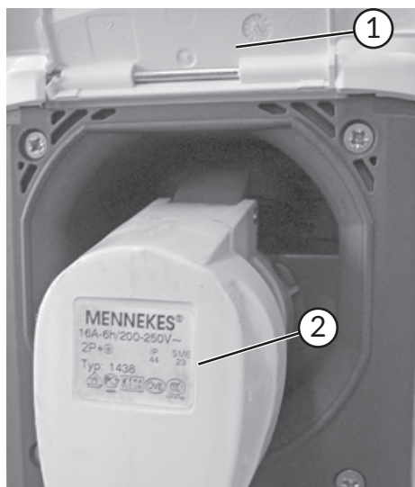
Connected 230V hook up
