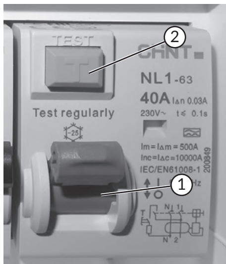
FI switch and test button
