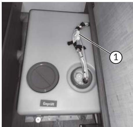
Switch for the water pump
