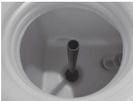
Overflow pipe of the fresh water tank
