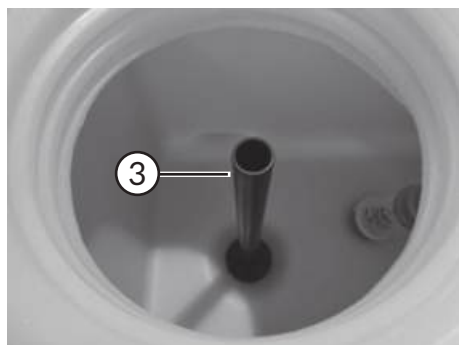
Overflow pipe on the fresh water tank
