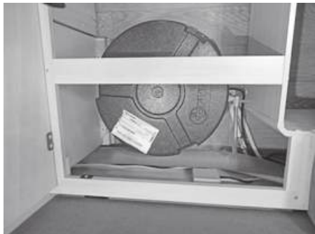
Boiler with drain valve
