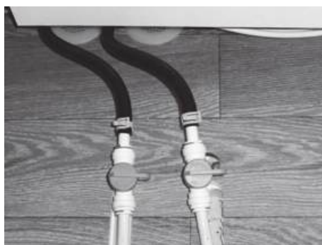
Valves in closed position
