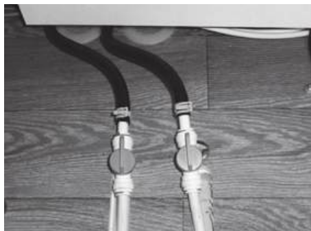
Valves in open position
